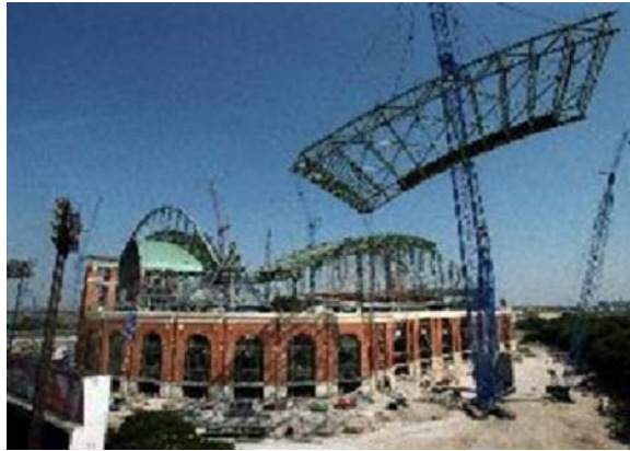
Figure 19.3 Stadium Construction Before Collapse
