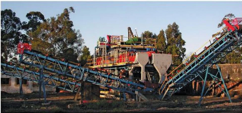
FIGURE 2.17 Mobile wash plant with 100 t/h feed capacity in South Africa
