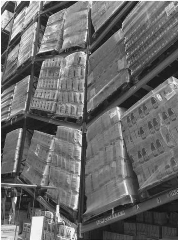
FIGURE 15.3 Partial rack collapse (courtesy of Nene)
