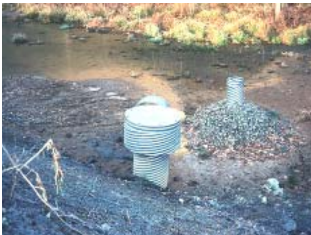
Temporary sediment trapping device attached to a riser assembly.
