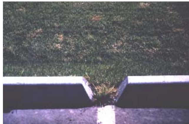
A clogged curb cut impedes flow entering the biofiltration system. A better design would have a wider opening with a small vertical drop to prevent sediment clogging of the opening.
