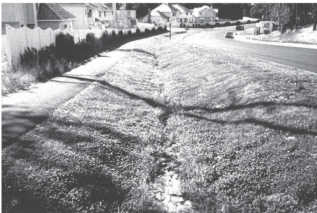
Sediment accumulation in a biofiltration facility reduces the effectiveness of that facility in removing pollutants. This swale is in need of maintenance to reestablish desired water quality control conditions.
