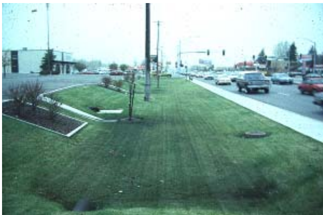
Well maintained biofiltration swale serving a commercial development. There is some evidence of oil staining of the vegetation.
