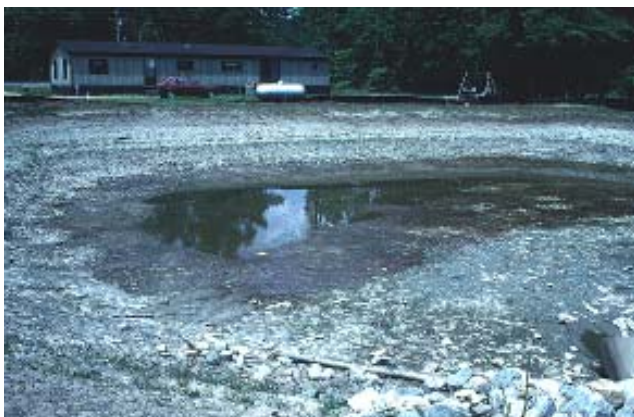
Excessive silt-clay sediments have clogged the basin floor causing this infiltration basin to fail.
