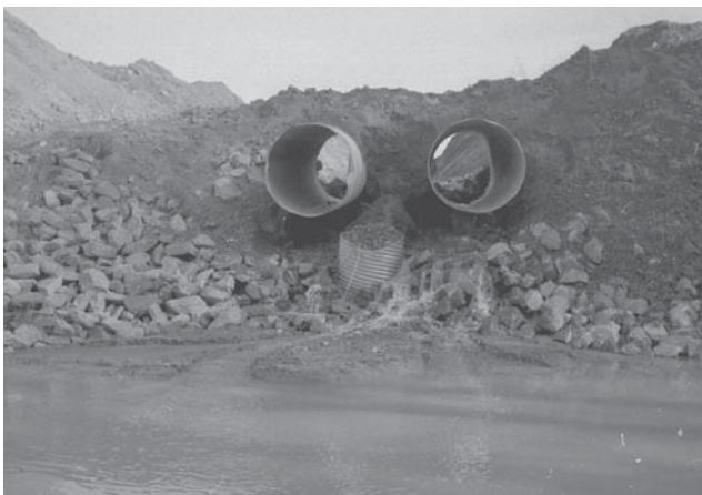
Water piping around a barrel. The water is flowing with considerable velocity.
