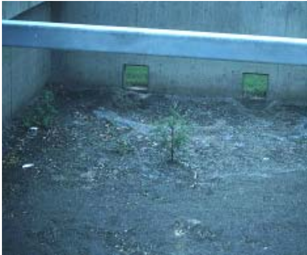
Evidence of scour at the entrance to the filtration chamber from the sedimentation chamber. The connecting areas between chambers should be protected with a nonerosive material, such as stone or a splash pad.
