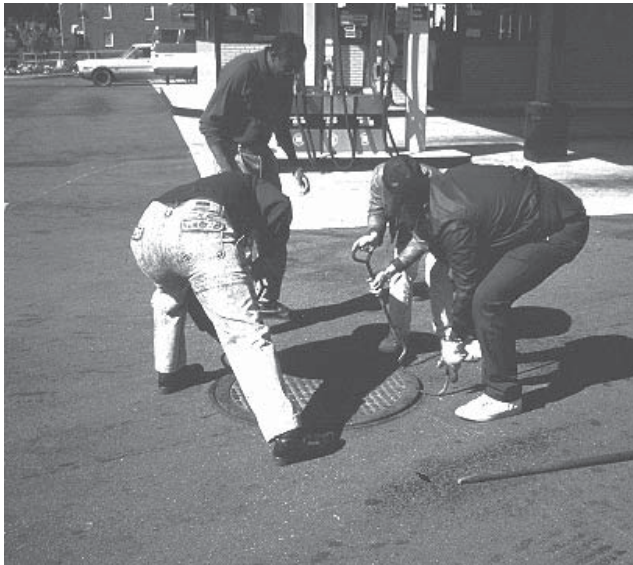
Inspectors lifting a manhole cover of a Washington, DC sand filter. Care must be taken in cover removal and replacement.
