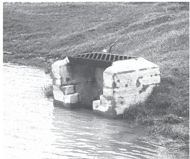
Broken up outlet structure. Having the grate on top doesn't really provide any factor of safety.
