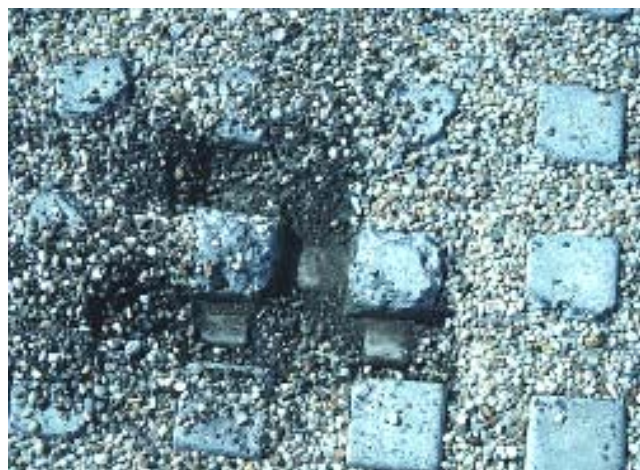
Lattice block infiltration system at a commercial parking lot. The open areas are filled with pea gravel to provide support for shoe heels.
