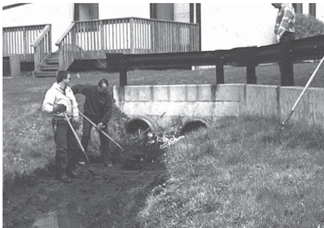
Removal of debris from the entrance of an outlet structure in a detention facility.
