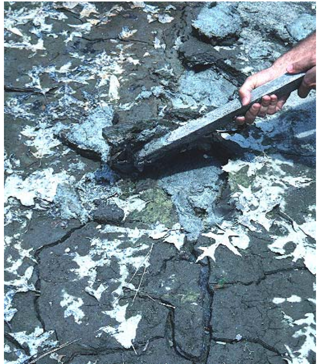
Close up sediments clogging an infiltration basin. Silt and clay sediments are the greatest concern since they can seal the basin/soil interface area.
