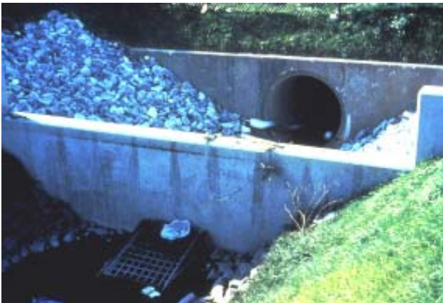
Extended detention facility where water quality is provided by the small orifice at the bottom of the weir. Maintenance should be mainly concerned with keeping the grate unclogged.
