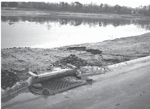
Example of clogged inlet causing erosion when water overflowed onto vegetated areas adjacent to a stormwater pond.
