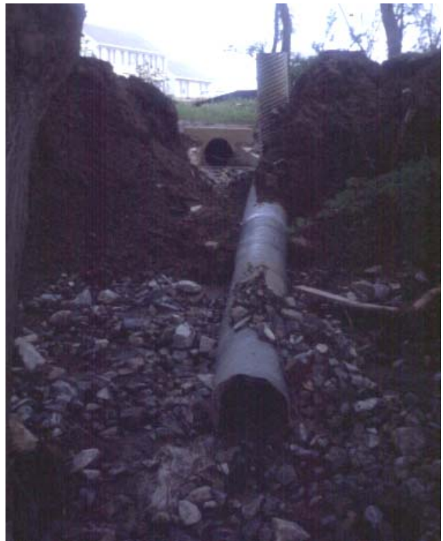
Example of a pond failure due to piping adjacent to the principal spillway.
