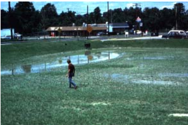
Standing water in a dry detention basin caused by a blocked outlet or bottom slopes which are too flat.
