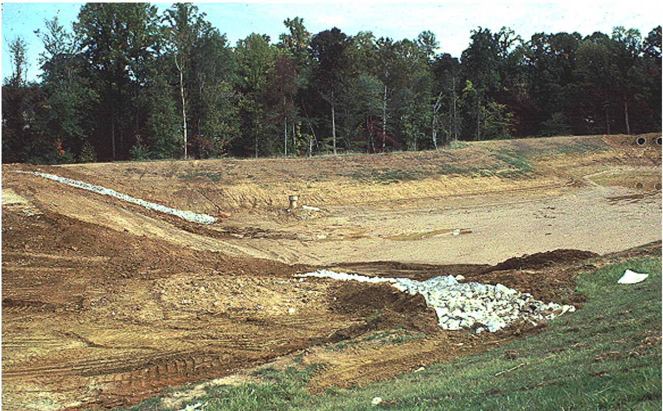
Sediment from construction activities can quickly clog an infiltration basin.
