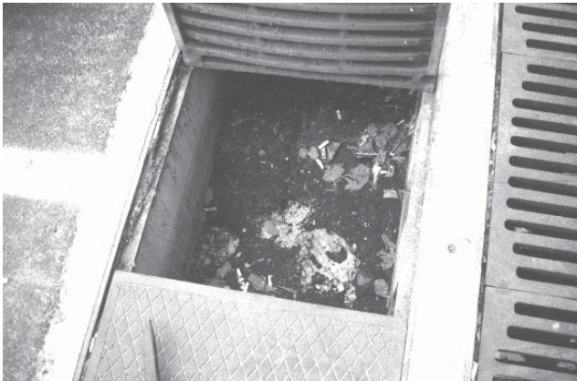
Sand filter showing trapped oils and greases.
