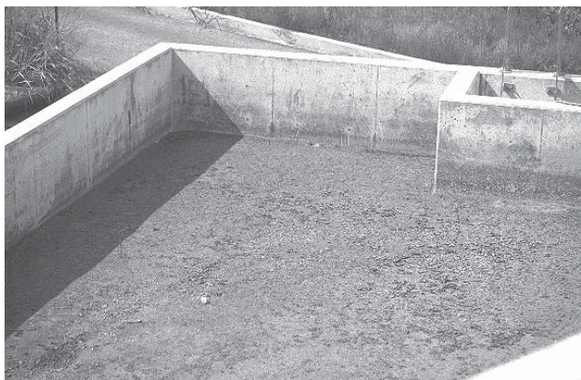
Filtration chamber of an Austin sand filter showing overflow spillway. The sand media needs to be inspected regularly to determine if design permeabilities are reduced.
