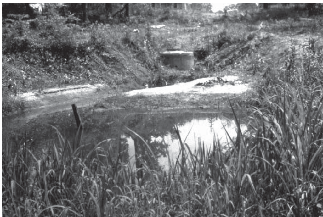
Lack of access prevents maintenance.
