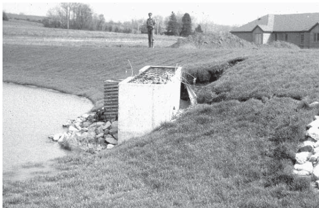
Erosion around the outlet structure of a stormwater management pond.
