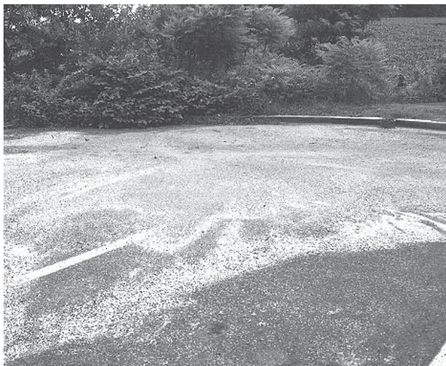
Porous paved parking lot clogged due to excess sediment on parking surface.
