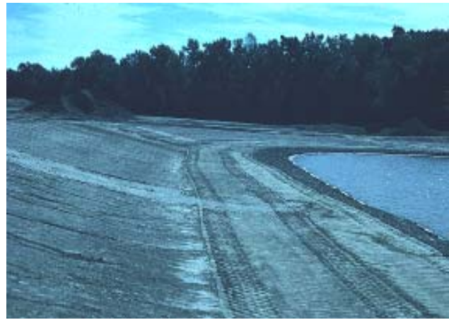
Pond under construction. Reverse slope bench above waterline and shallow slope in shallow water areas.
