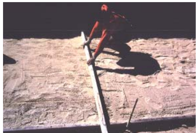
Foundation grade being established prior to placement of concrete floor of the filtration facility.
