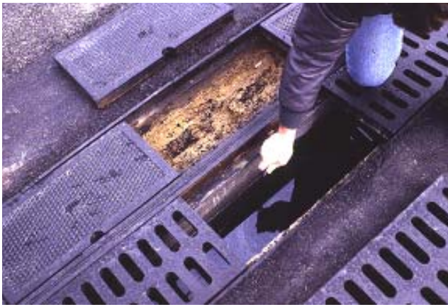
Sand Filtration Facility
