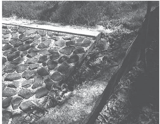
Erosion behind the grouted riprap wingwall will eventually cause failure of the riprap, which will increase sediment loadings downstream negating the BMP's benefit.
