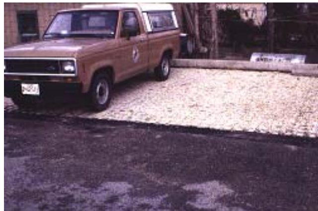
Lattice block infiltration provided at a parking lot.
