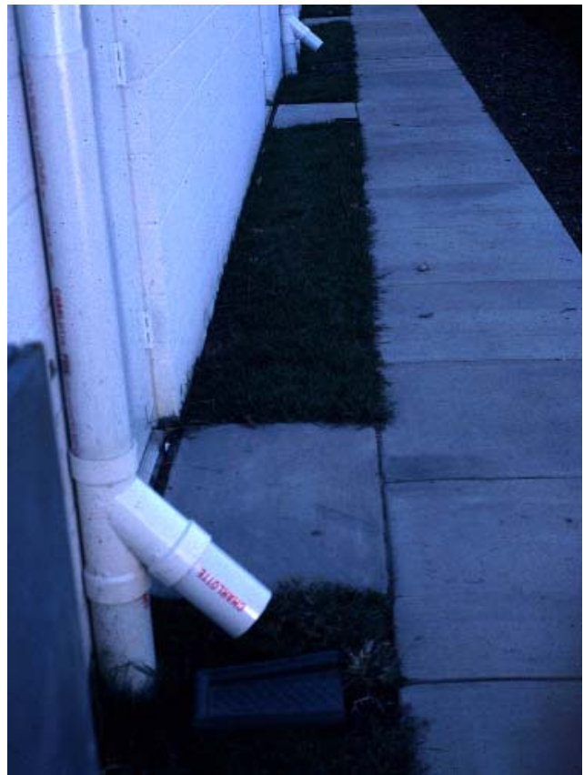
Completed drywell showing overflow device: note total site utilization but also the lack of observation wells.
