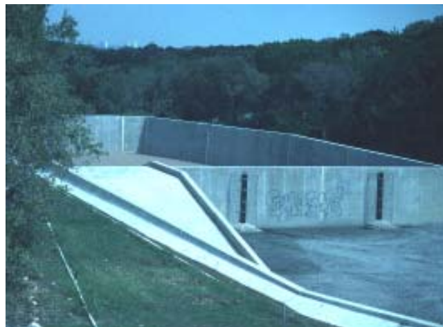
City of Austin sand filter for new highway construction. The chamber in the foreground is the sedimentation chamber, the filtration chamber is in the background.
