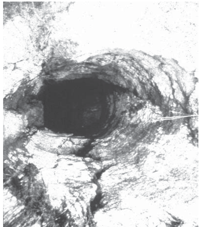
Solution pipe sinkhole in the bottom of an infiltration system.
