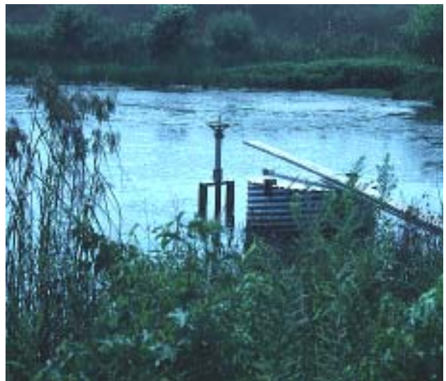
Gate valve for a stormwater management pond. When maintenance inspections are done, the valve should be operated and lubricated to ensure proper function.
