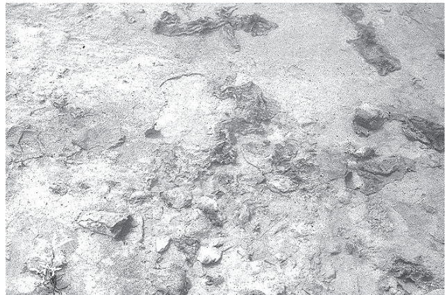
Algae on an infiltration basin floor has caused failure of the facility by preventing infiltration of stormwater.
