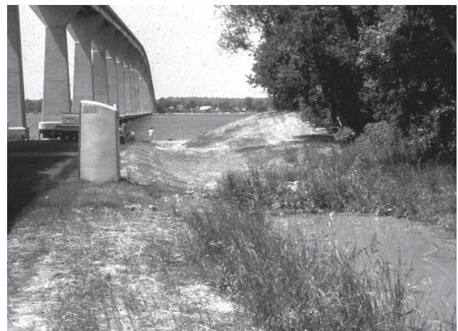
Clogged infiltration swale. The individual swale blocks must be dewatered before accumulated sediments are removed.
