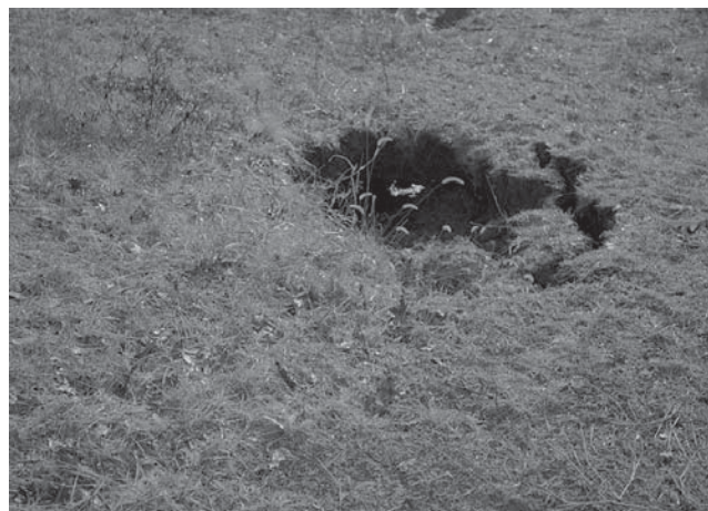
Example of a hole on a stormwater pond embankment. This indicates two concerns: (1) watch where you walk; and (2) the pond has serious problems with piping around the barrel assembly. If you see this, get assistance.
