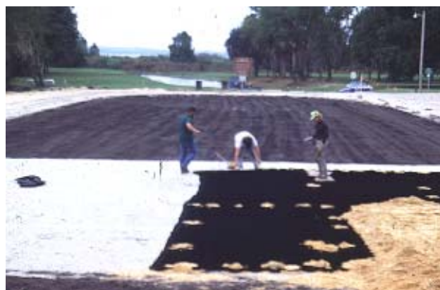
Geoweb fabric being installed and filled with sand before sod is added to create grass parking.
