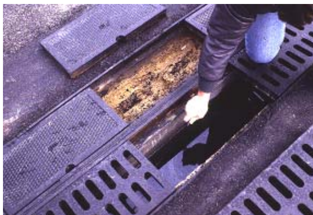
Delaware sand filter showing both the sedimentation and filtration chambers. The sedimentation chamber is permanently filled with water to prevent resuspension of the accumulated sediments.
