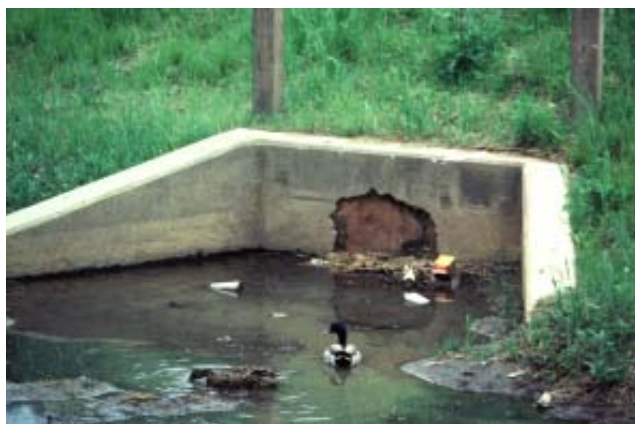
Partially clogged outlet at a detention basin due to not inspecting or maintaining the facility.
