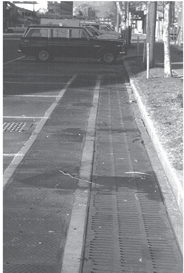
Waste oil was dumped in this Delaware sand filter and sealed the filter media almost immediately. The top several inches of sand had to be replaced. On the good side, if the filter were not present, the oil would have been discharged on the community beach.
