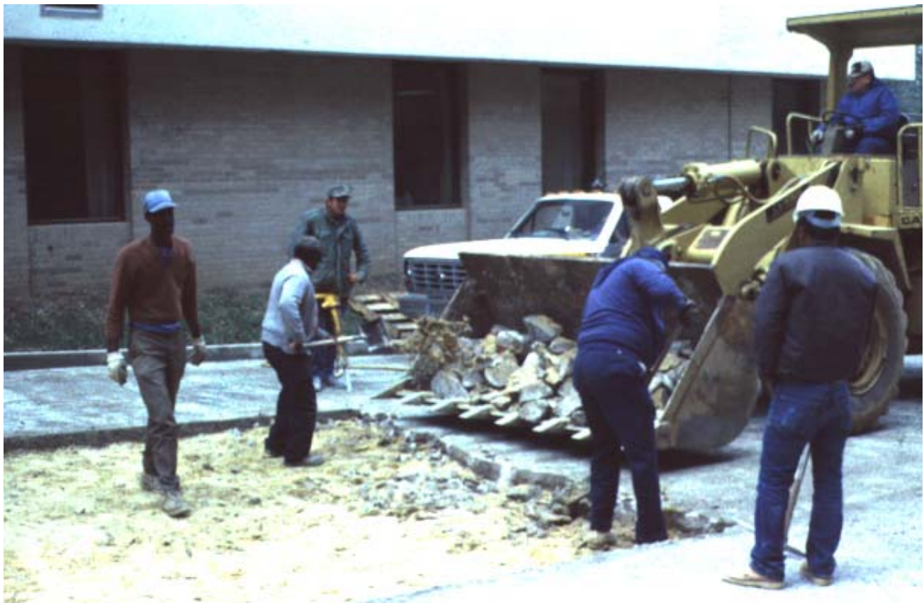
Improper batching at Florida Dept. of Environmental Protection parking lot necessitated replacement of pervious concrete section.
