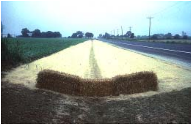
Swale biofilter having erosion control matting installed prior to permanent vegetative stabilization.
