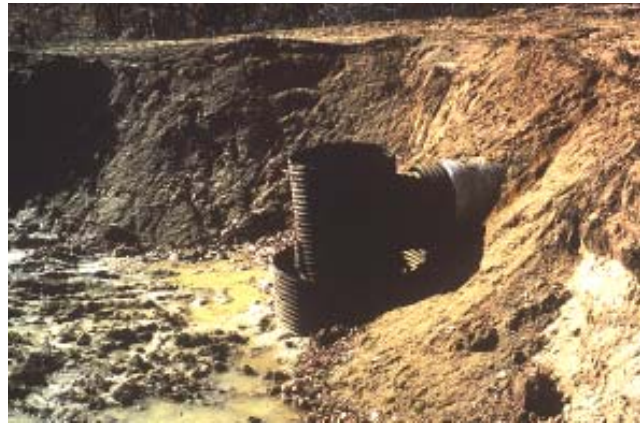
Barrel/riser assembly installed upside down demonstrating a lack of understanding by the contractor and lack of inspection oversight
