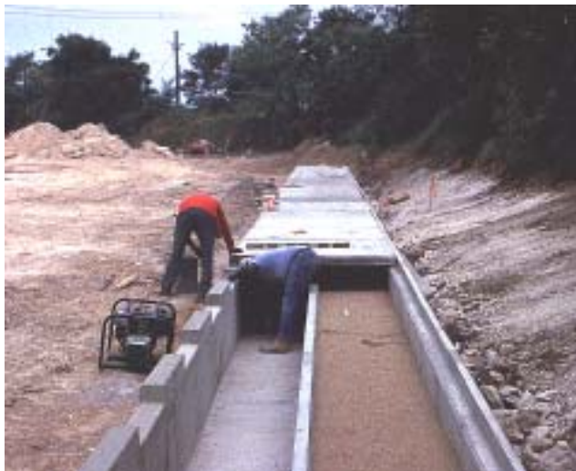
City of Alexandria variation of the Delaware sand filter using prefabricated concrete tops for the filter.
