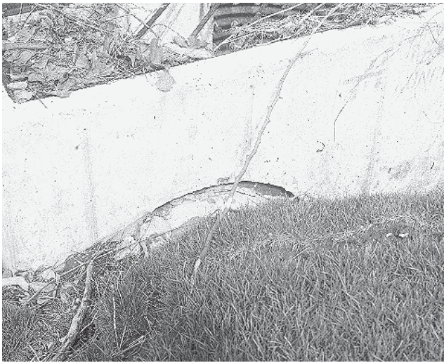
Leakage around the barrel and riser assembly. This could cause piping of water adjacent to the barrel which would jeopardize the structural strength of the facility.
