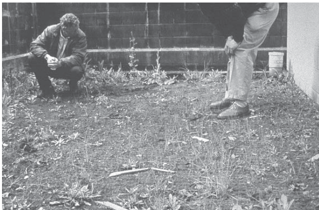
Sand filter in Auckland, New Zealand. The sand filter serves a commercial parking lot. Vegetation growing in the filtration chamber may indicate a need for maintenance.
