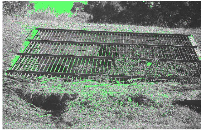
Example of debris which is beginning to clog the outlet structure of a detention facility.
