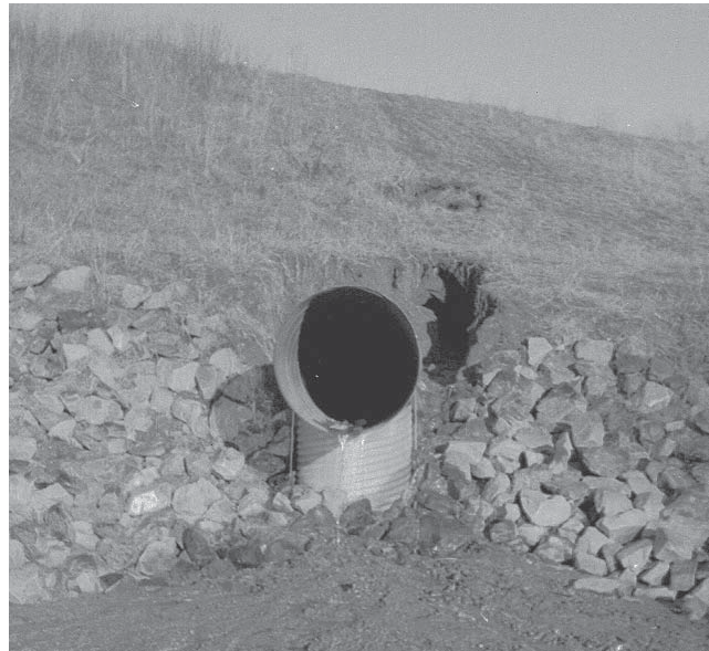
This may be as bad as it gets. This retention facility was in a state of failure. The embankment had to be breached and completely rebuilt. The problem resulted from seepage around the barrel causing embankment soil to move with the flow of water. This failure resulted from poor construction.
