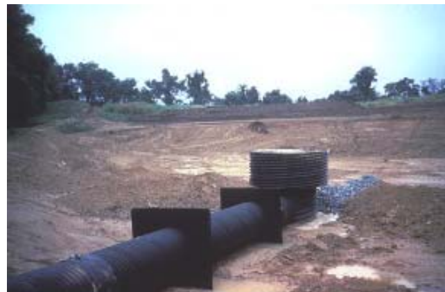
Anti-seep collars, barrel, and riser assembly for a stormwater management detention basin.
