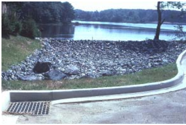
Completed infiltration basin; note the lack of pretreatment measures prior to runoff entry into the facility.
