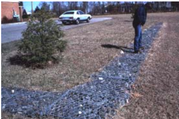
Two infiltration trenches on the same site. The value of the vegetative buffer strip can clearly be seen.
