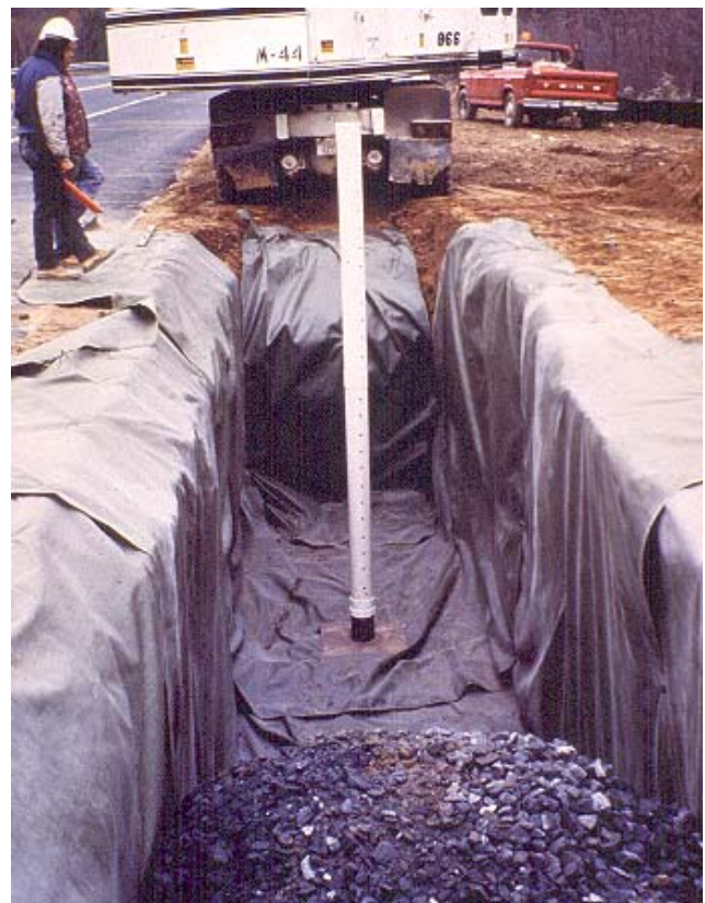
Infiltration trench showing the observation well, foot plate, and filter fabric side walls before placement of the aggregate.
