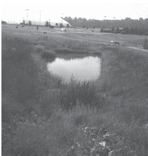
Example of a failed infiltration basin caused by clogging and not seasonal or mounded water table. The basin should be pumped of water and allowed to dry out before sediment is removed.
