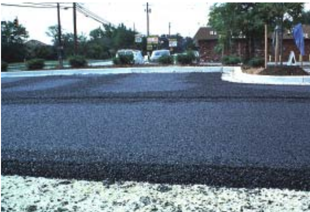
Porous paving being installed showing the porous asphalt course and the filter course.
